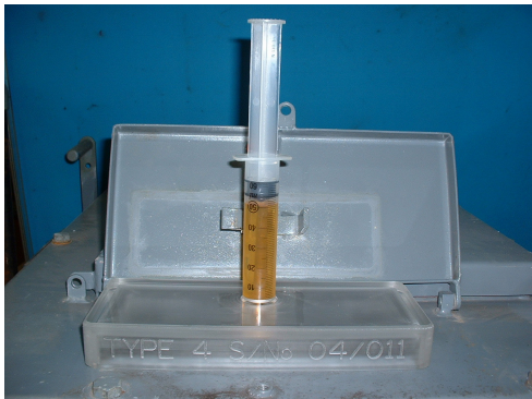
Diagram above: Test Access Cover Plate and Sample Kit Fitted on a Long and Crawford T3GF3 Ring Main Unit
